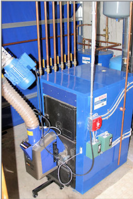
A Modern Wood Pellet Boiler in a 4200 sq. ft. Maine Home
