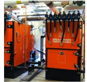
A biomass thermal system can provide hot air, water, and process heat
